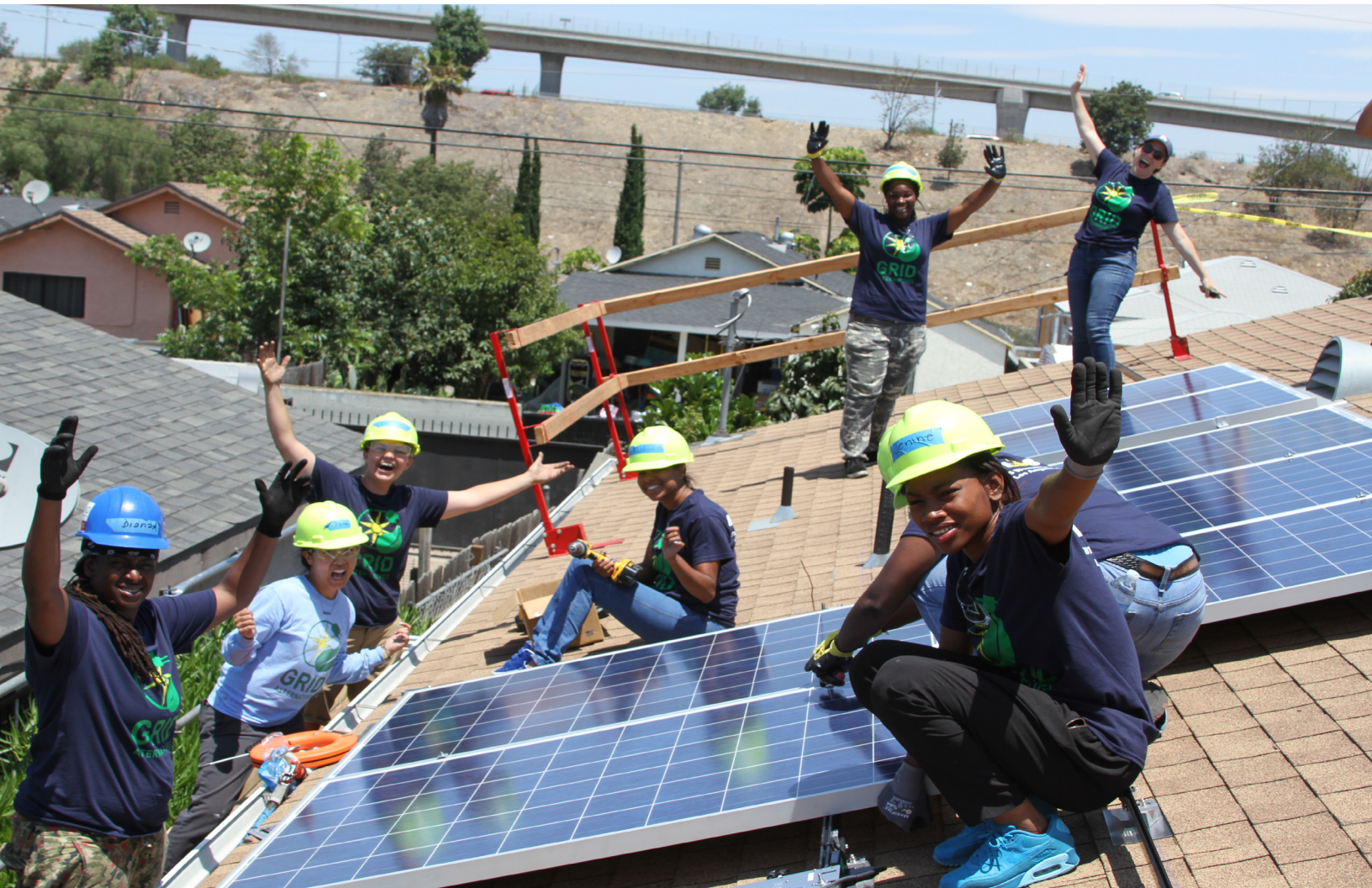
Team of workers from GRID Alternatives install solar panels on the rooftop of a Los Angeles house.
